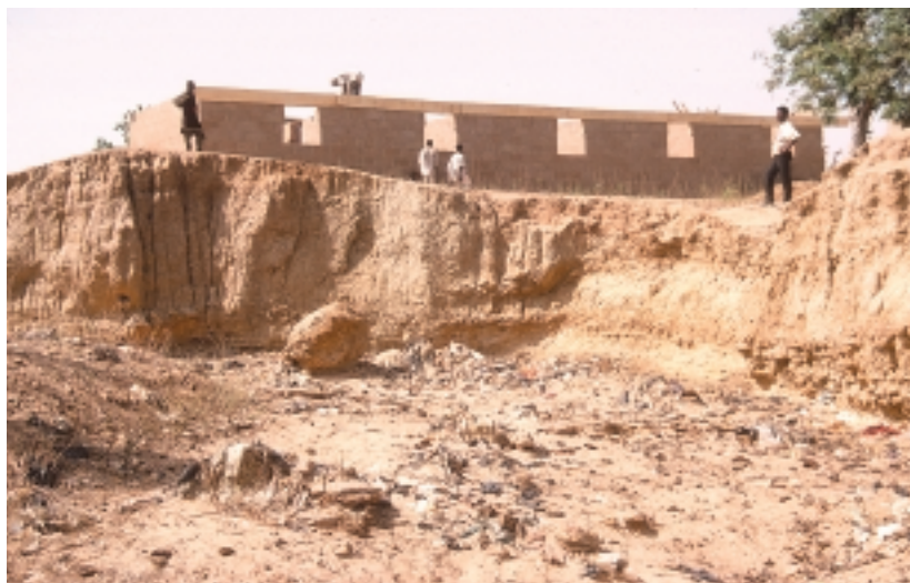
Photo 3: Close to an undercutting slope of a seasonal river a new building is under construction
