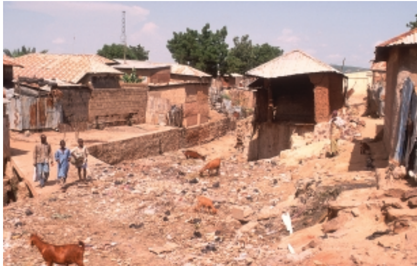
Photo 2: A flash flood damaged this house in the old town adjacent to a sewage gully (Photo: BALZEREK 2000)
