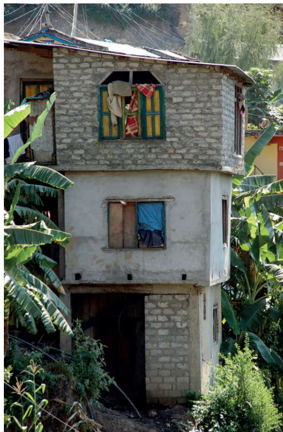
Photo 3: Partly framed Reinforced Concrete with soft storey and vertical irregularity (unsupported columns on upper floors) (Photo: J. ANHORN 2012)
