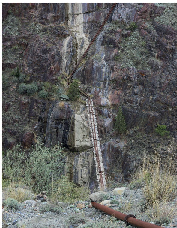
Photo 1: The bridge scheme for irrigation in Khaiadar and Tamareil, Minapin. (Photo: SPIES, April 2015)
