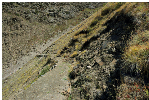
Photo 3: Blocked irrigation channel between Khu and Thobishen, Hopar area, due to land slumping triggered by free-grazing yaks. In the gully visible in the background of the picture, debris flows have destroyed parts of this channel that had been rehabilitated through a joint AKRSP-Caritas Switzerland project in 2013. (Photo: SPIES, September 2015)
